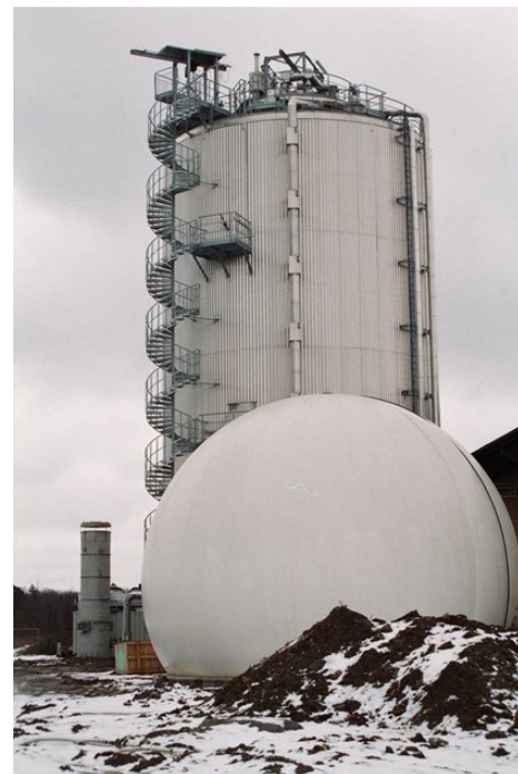
Figure 5. A DRANCO single phase silo reactor used to digest solid municipal waste in Germany (from www.tkm.sebe.eu ). Sphere in foreground is biogas storage.
