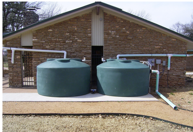
Figure 5: Rainwater harvesting system capable of capturing 2,200 gallons at the Xeriscape Gardens in Edmond, Oklahoma.
